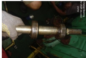
Gambar 1. 5 Shaft pompa sentrifugal.
